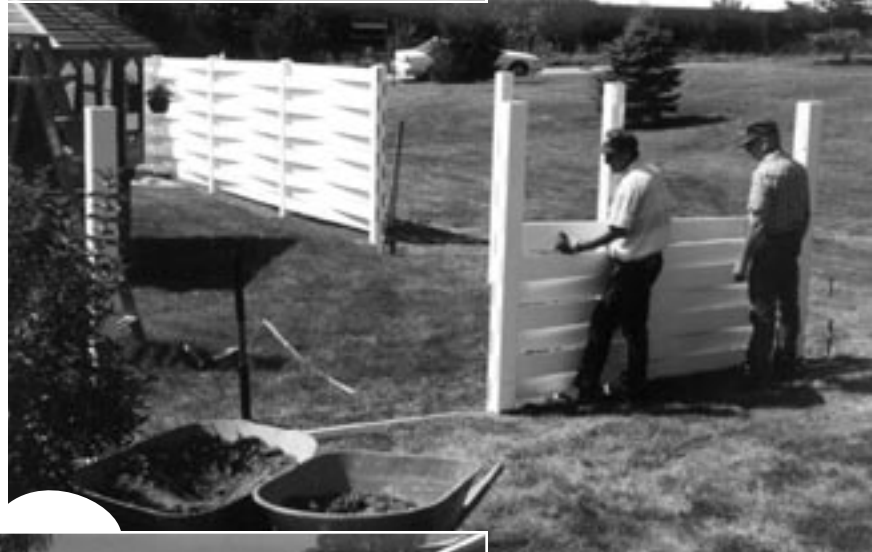
Prebuilt fence sections or horizontals are then mounted to or through the routed posts.
